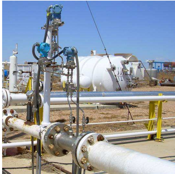
Fig 5. 4", 0.6 beta ratio Venturi meter installed in the CEESI wet natural gas loop.
