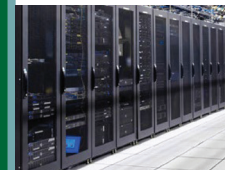
IOT Monitoring System
